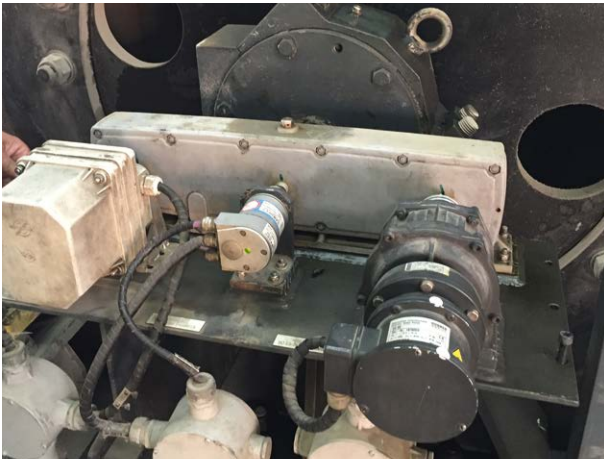
Before: Distribution gear with mechanical cam limit switch, absolute encoder and mechanical overspeed switch
