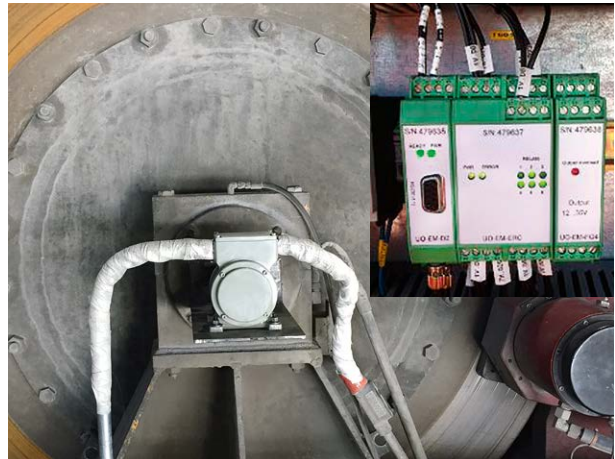
After: Direct mounted U-ONE basic unit with electronic modules in the switchboard
